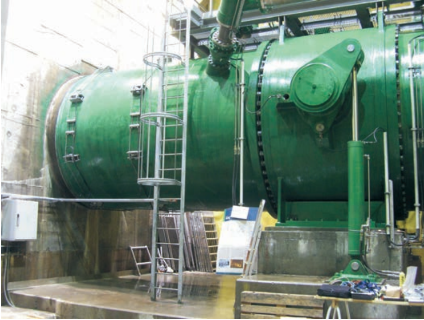
Installation in Iceland
